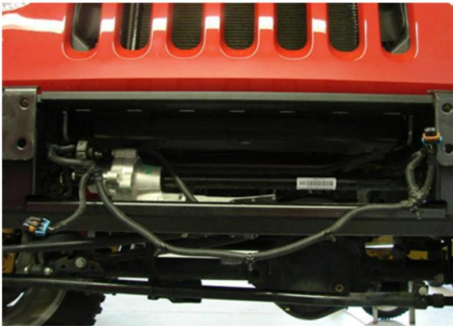
Original Wiring Position
